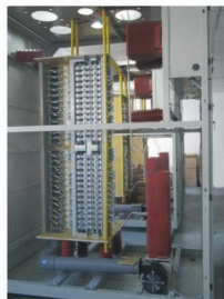
High voltage static Var compensator
